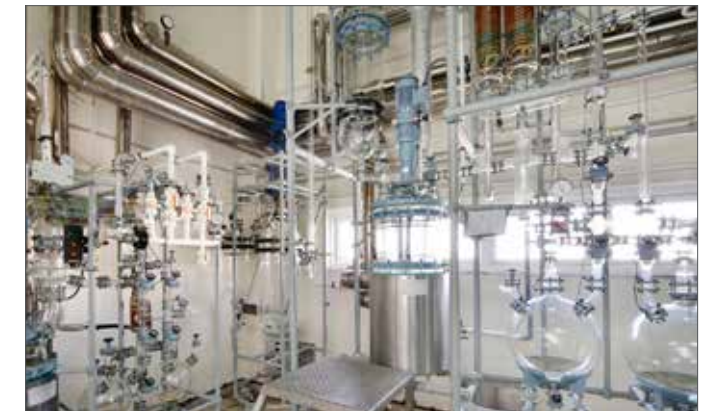
HIGH PURITY PROCESS PIPING
